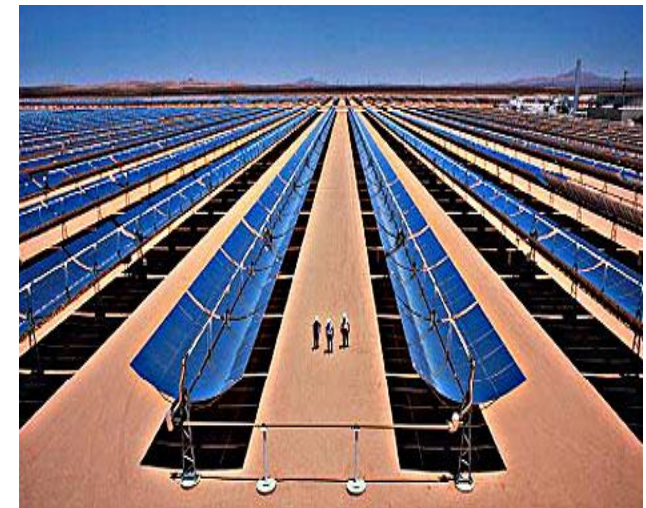
Acciona Solar thermal power plant located south of Las Vegas
